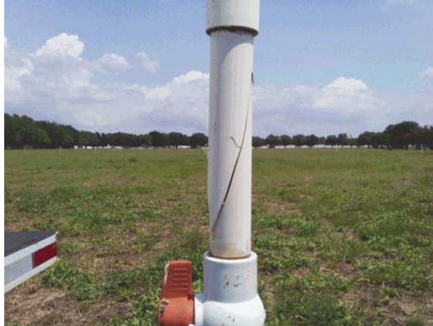
Typical sprayfield sprinkler head damage. 54 sprayfield repairs have been recorded in the past two months.
