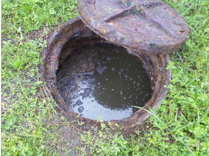
Sewer back up caused by failed manhole.
