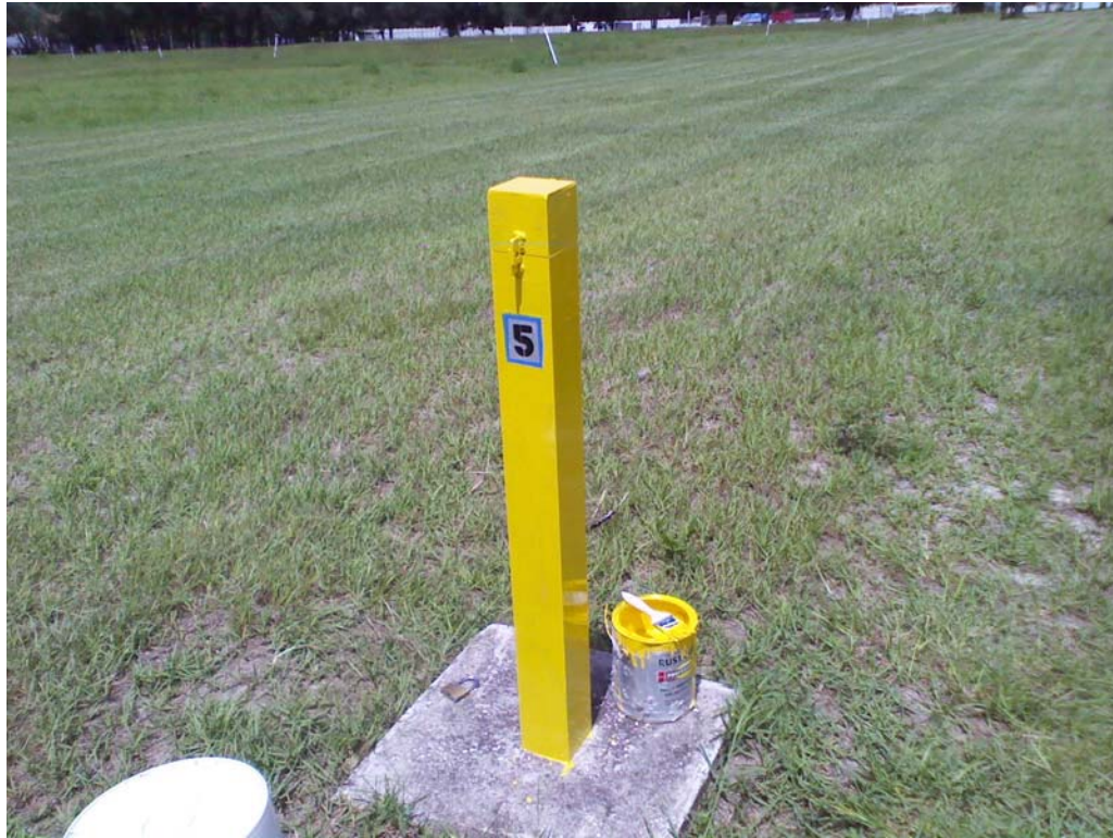
Monitoring well location after being maintained.
