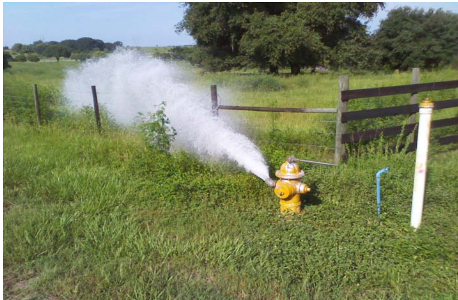
Routine flushing of fire hydrants.
