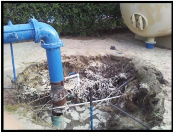
Water main break at Jacob WTP.
