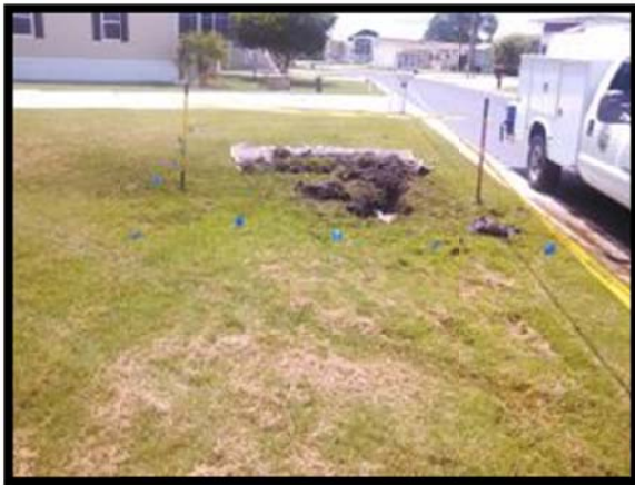
Leak on Island View Circle
