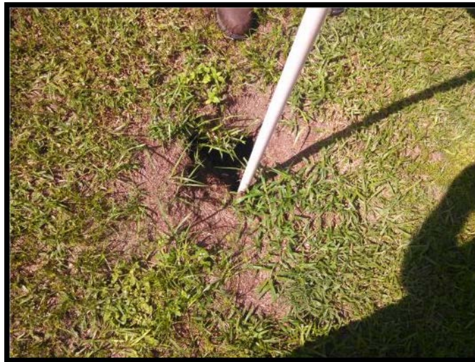
Sinkhole on Greenleaf Rd.
