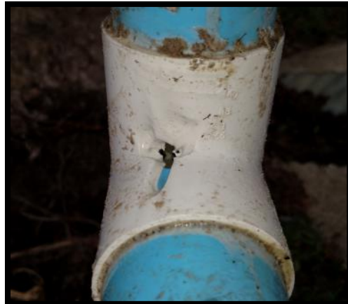
Hole in service line.
