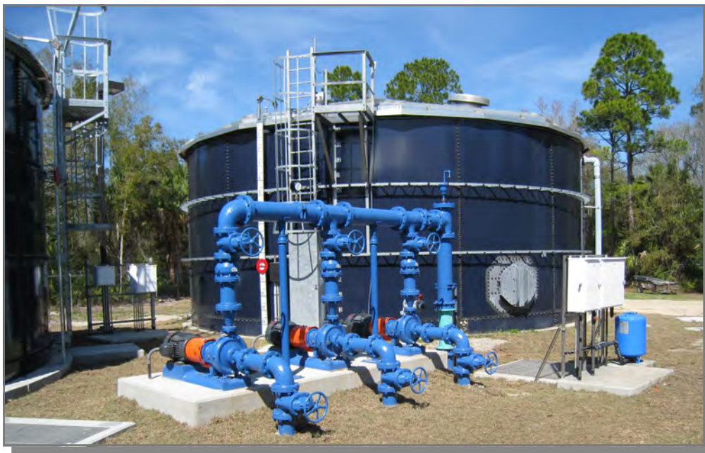
SRF WATER TREATMENT PLANT, YANKEETOWN, FLORIDA
