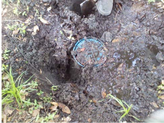
1 st water leak location after water was shut down.
