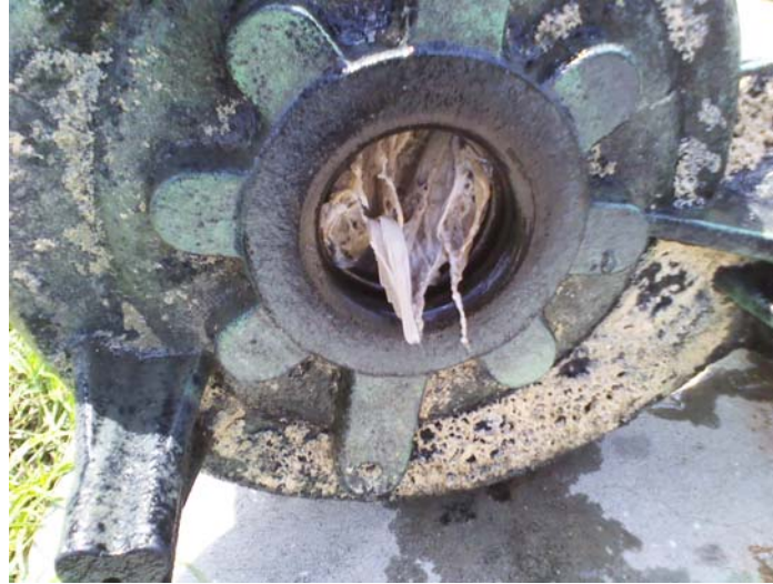
Typical clog on a lift station pump.
