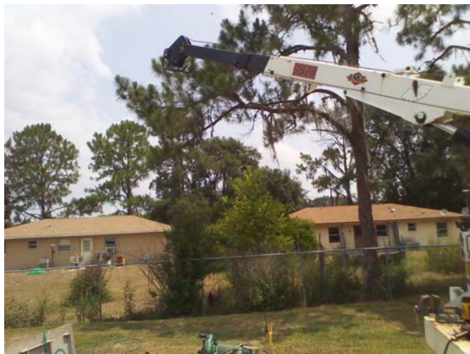
Lift station pump being pulled for routine maintenance
