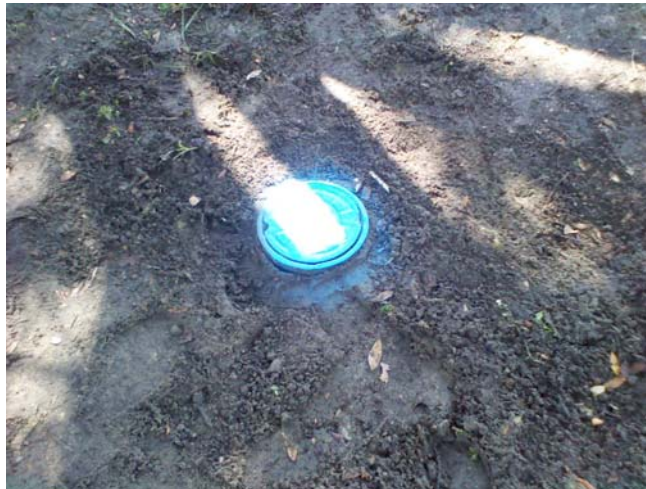
1 st area leak after repair was completed and water was restored.
