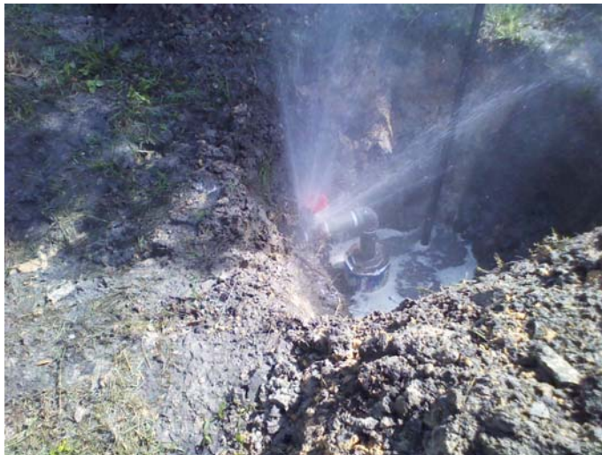
Main line blowout on 1 st street on Polk City system.
