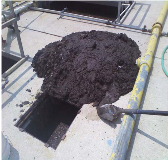
Cleaning tank at Mt. Olive WWTP
