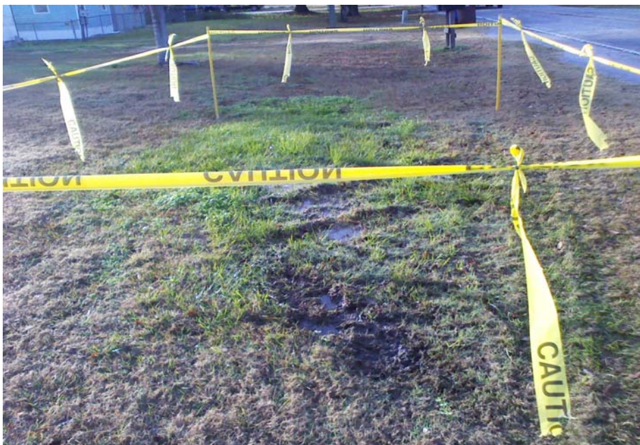
Water main leak on Berkley Rd.
