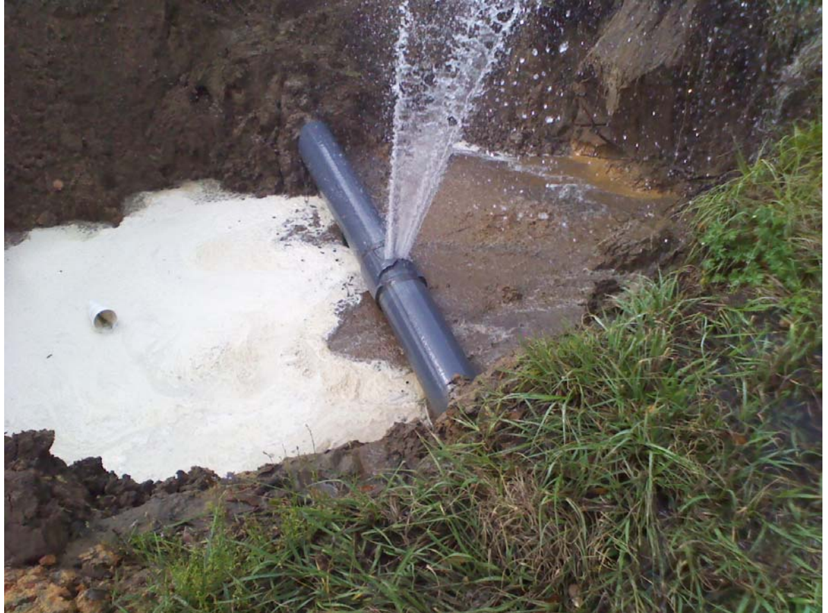
Cardinal Hill reclaimed water line break.
