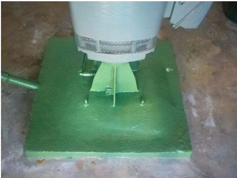
CommonWealth well pump out of service.
