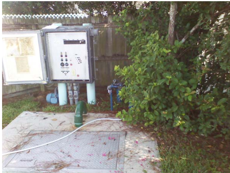
Old lift station set to be replaced as part of new project.
