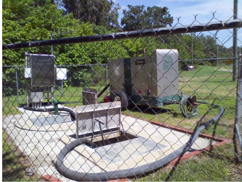
Lift Station #1 (Brooks Ln.) with diesel back up pump.
