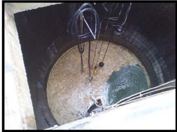
Typical amount of grease found in liftstations.
