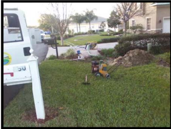
Leak on Bay Berry Dr.
