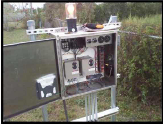
Electrical panel at liftstation #11
