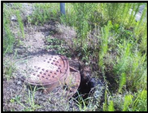
Top broken off of man hole.
