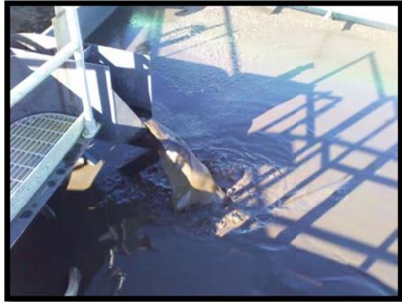
Wasting Activated Sludge at Cardinal Hill.
