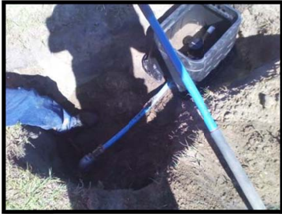
Typical meter installation.
