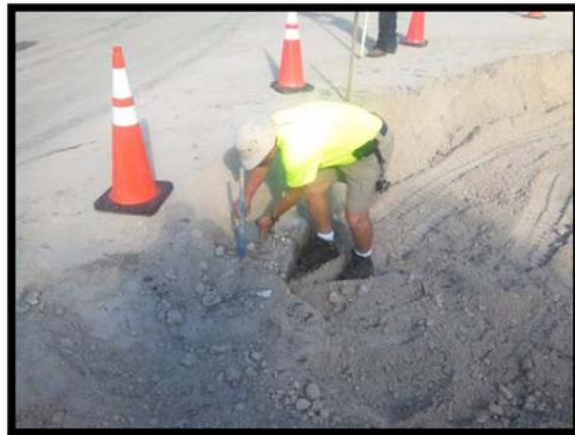
Valves on SR 33.
