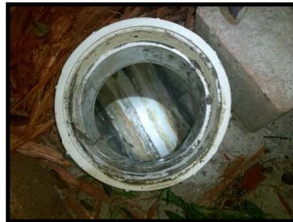
Typical customer cleanout.
