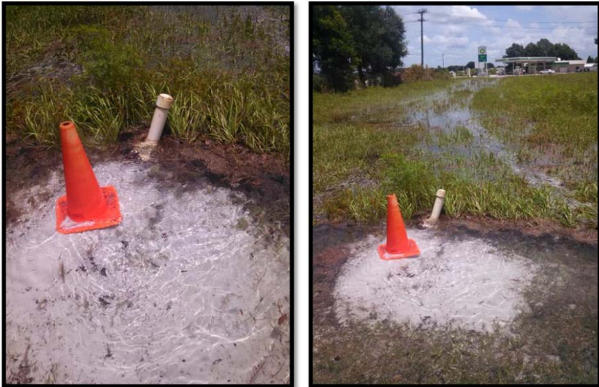
Initial leak from 2 ½ inch water line on Fountain Park irrigation system.
