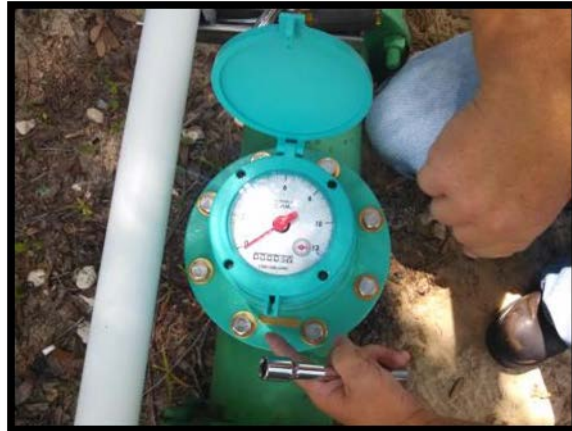
New flowmeter at Commonwealth WTP.
