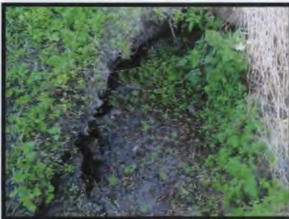
Depression found over sewer line.
